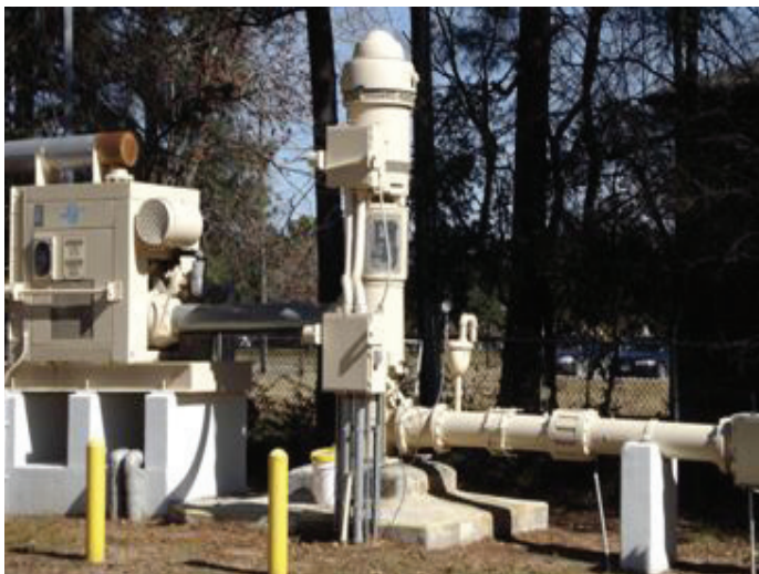
Deep well vertical pump and 400 HP motor at Well-1 Pumping Facility.
